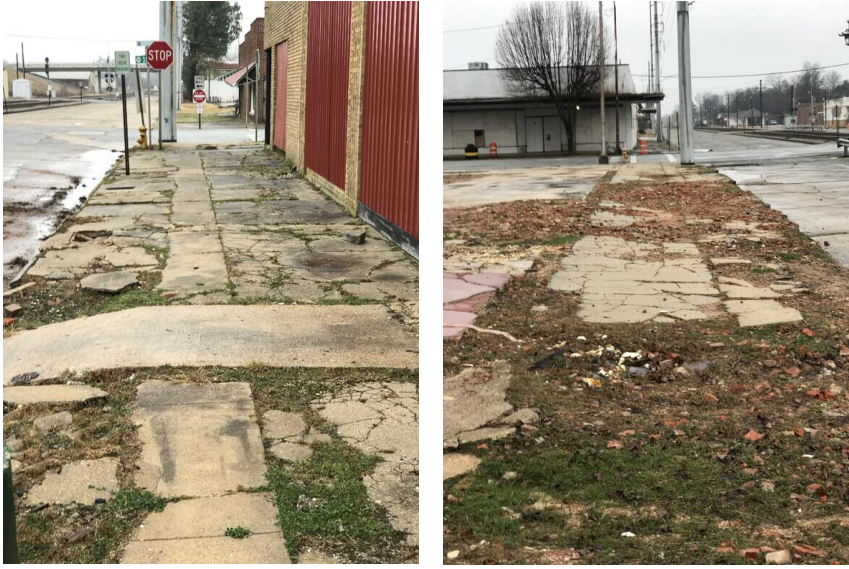
Current sidewalk condition on 4 th and Main in downtown Pine Bluff
